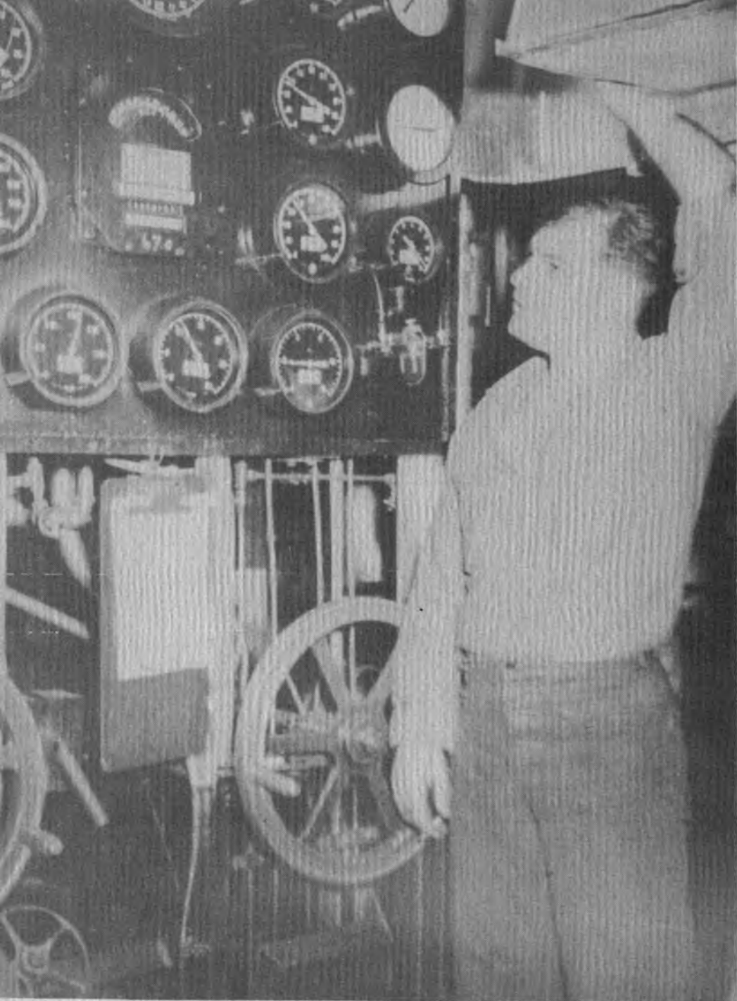
Engine Room, Main Control
